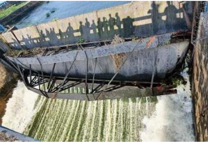
Fig.3(a): GATE DAMAGE
